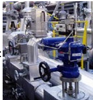
STEAM PRESSURE REDUCING STATION
